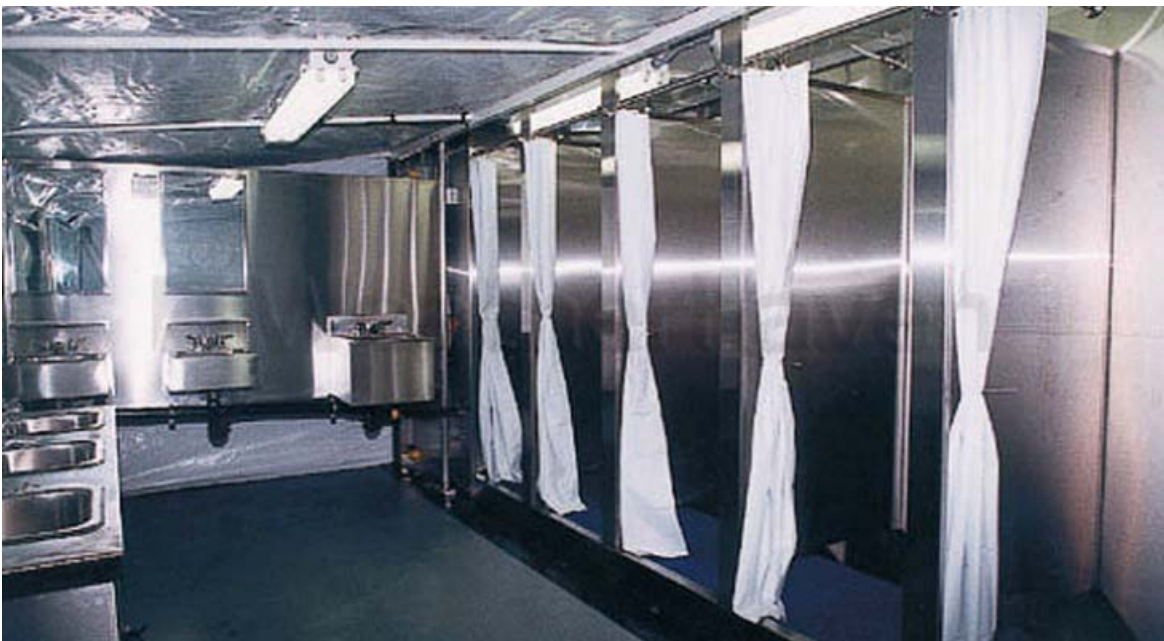
Figure 24. Weatherhaven Ablution System (Weatherhaven, 2011c)
