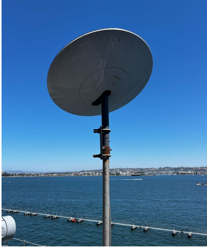
Figure 3. Starlink Terminal Mounted on Port Quarter
